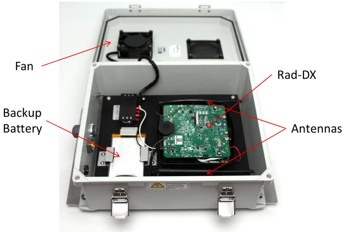
Figure 5: Inside the NEMA Enclosure
