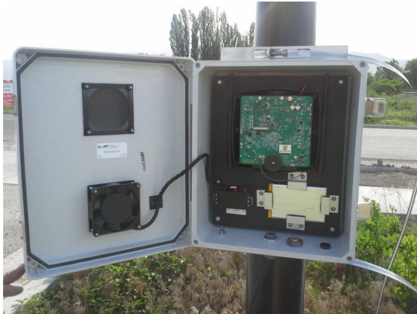
Figure 3 - Rad-DX NEMA Enclosure on Pole
